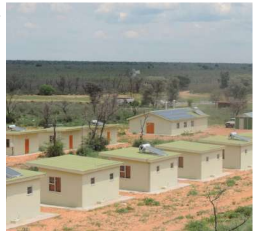
Construction of the Law Enforcement Training centre at Waterberg has commenced with funds through the Game Products Trust Fund (GPTF)
