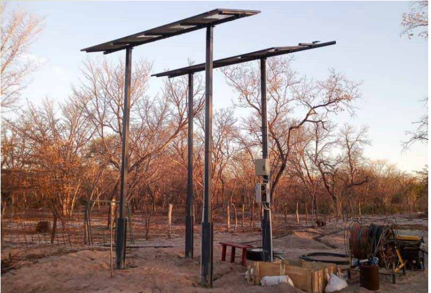
Rehabilitation of the converted borehole from monitoring to a water supply borehole with pipeline extending to 23 kilometres.
